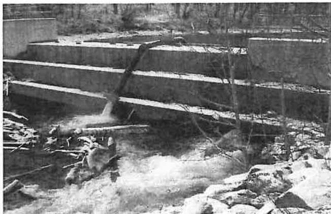
At right bottom, water flows from existing 24 inch pipe. In center is first of six 12-inch pipes that are now installed.
