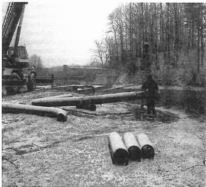
Worker cuts pipe to fit over Onota dam, in background. (Cuyler photo)
